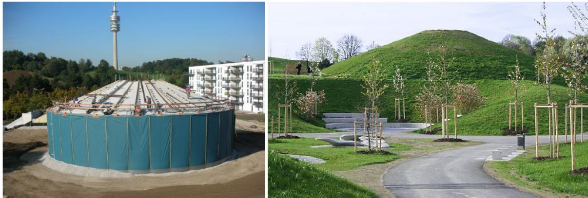
Figure 30 - TTES with 5,700 m 3 of water volume built from prefabricated concrete elements in Munich, Germany (in construction and finalized, Solites).
